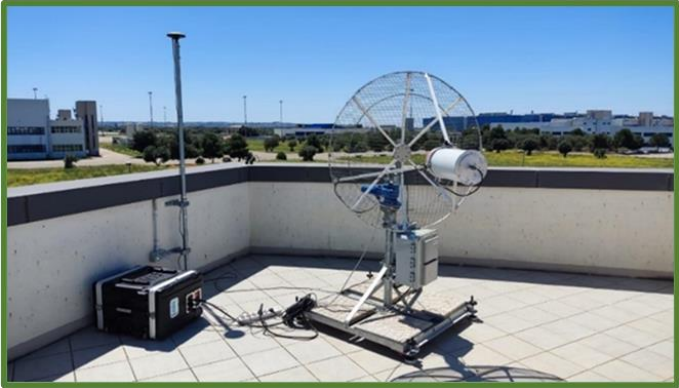
RFI monitoring station deployed at GATB on the roof of the control tower
