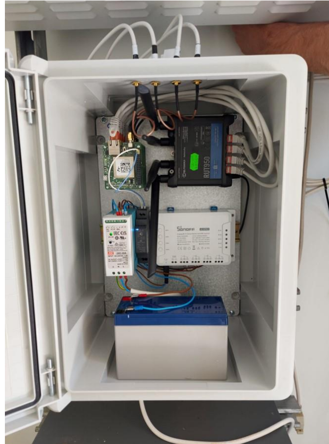
Box with GNSS receivers, 4G router, power supply and smart switch
